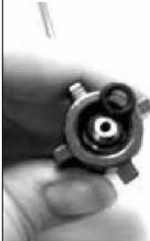
CO2 line to regulator
